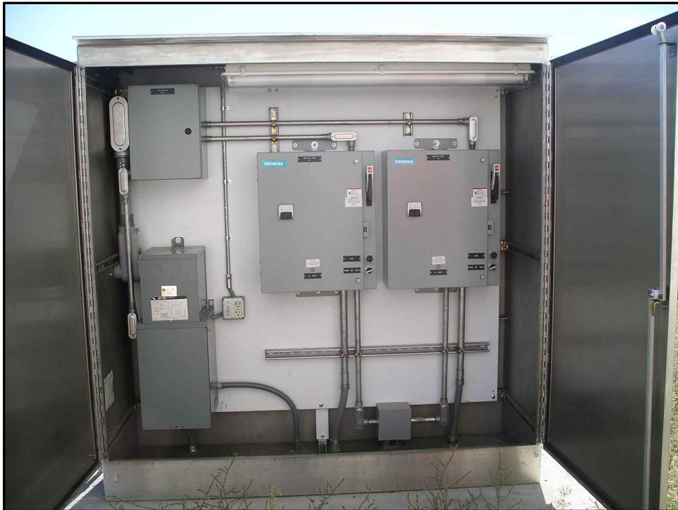
NORTH RESERVOIR BOOSTER PUMP NO 1 & NO 2 PANEL
