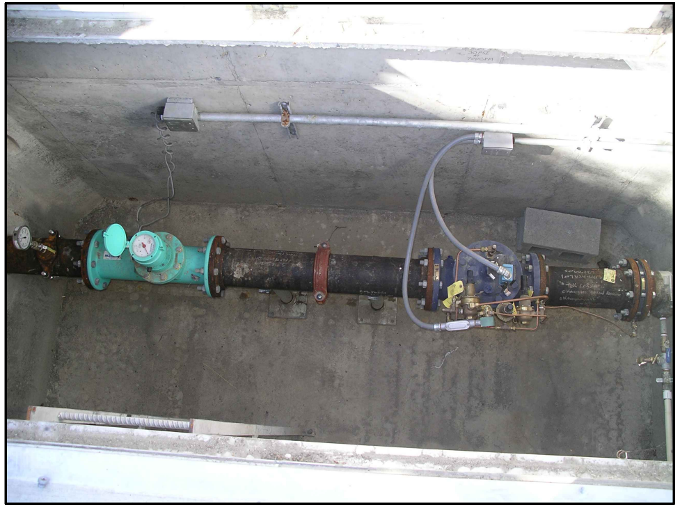
TRANSFER STATION VALVE & METERS (IN VAULT)
