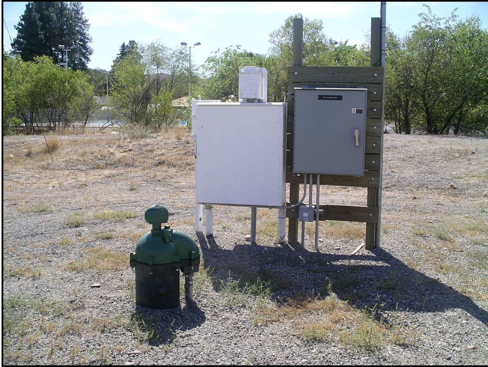
WELL NO 4 & TELEMTRY
