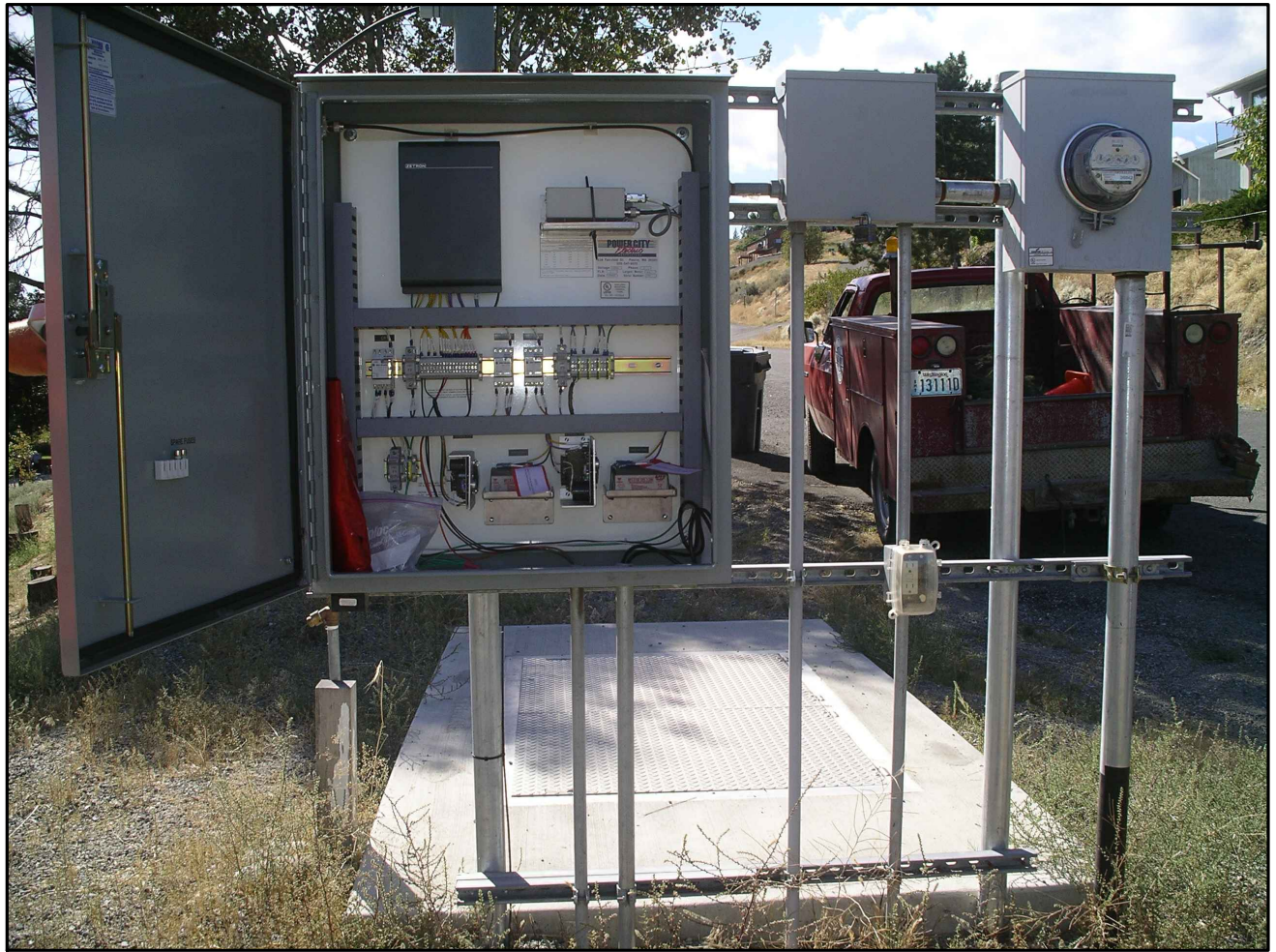
TRANSFER STATION TELEMETRY PANEL
