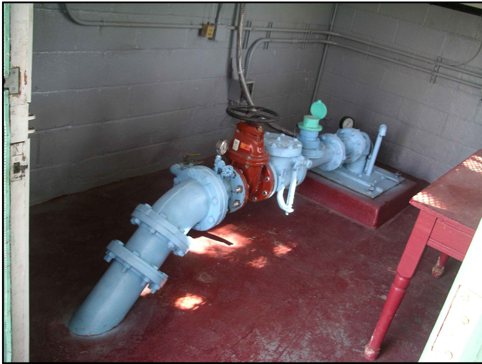
WELL HOUSE NO 2
