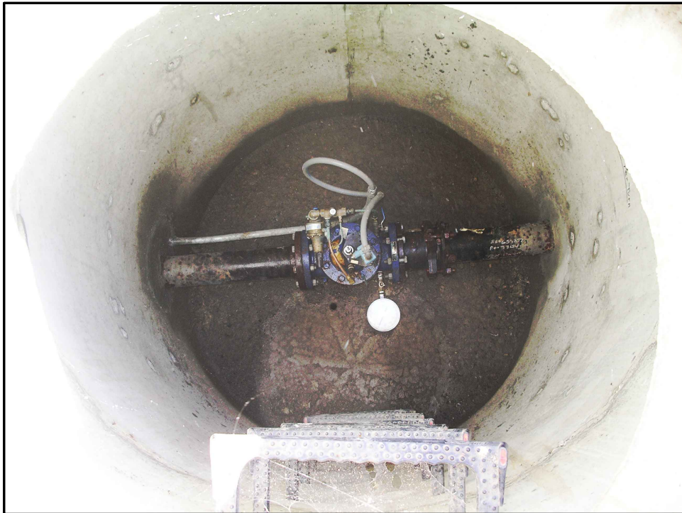
NORTH RESERVOIR BPS VALVE (IN VAULT)
