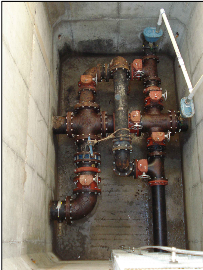
WEST RESERVOIR NO. 2 VALVES (IN VAULT)
