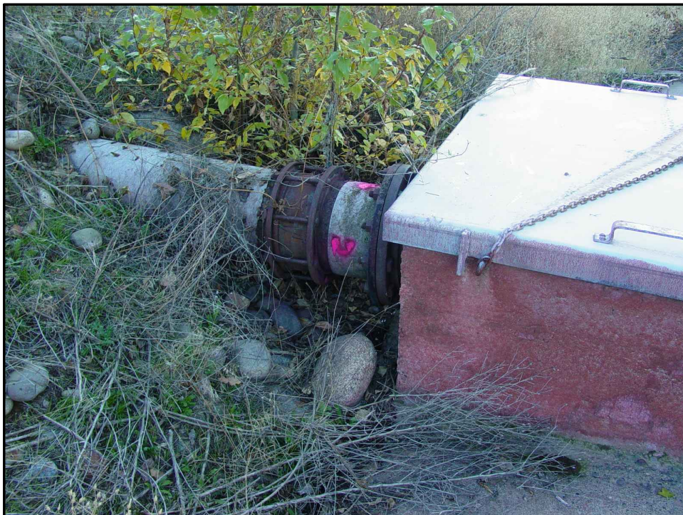
WATERCRESS SPRINGS RESERVOIR INLET PIPE
