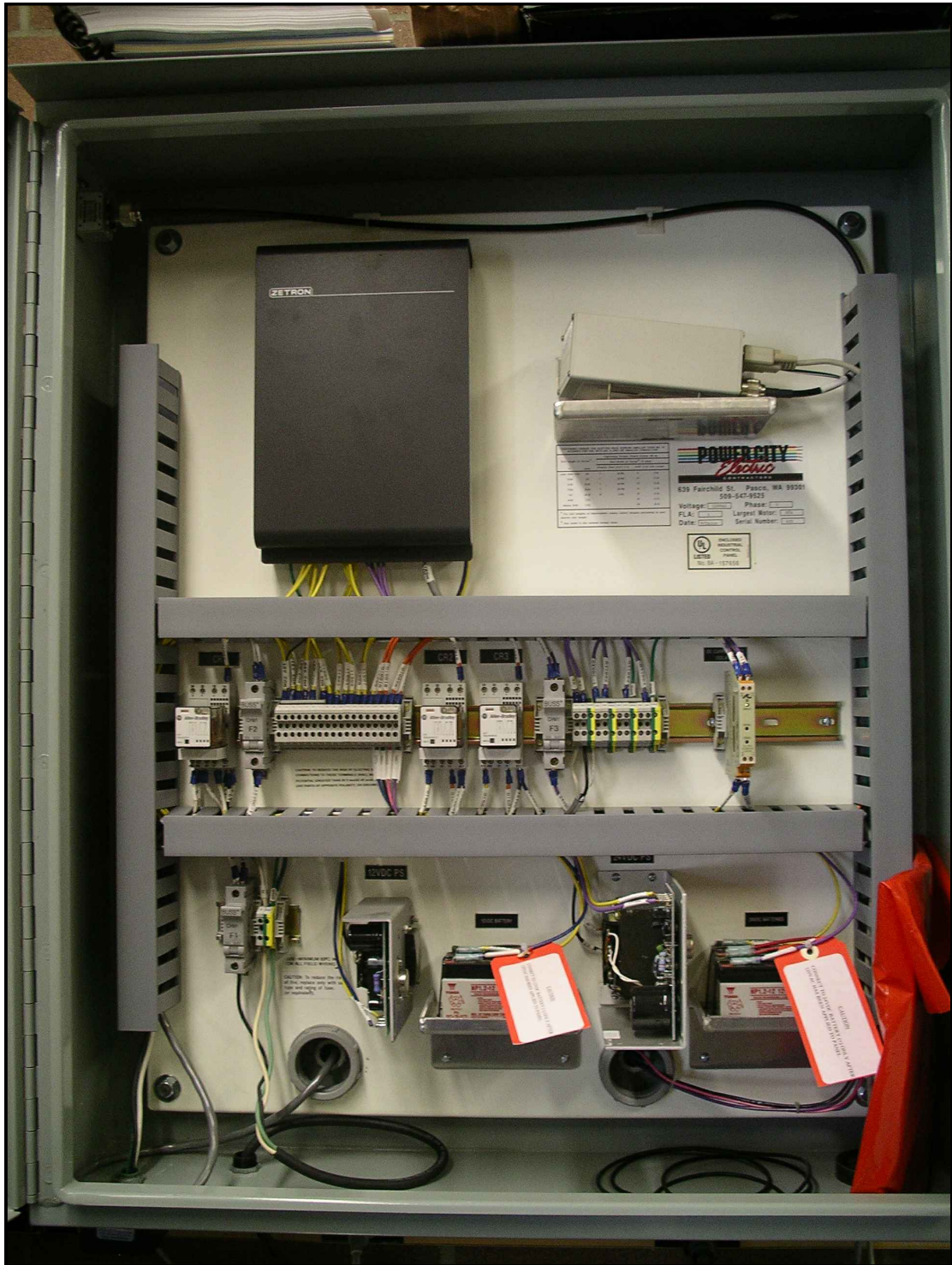
MASTER TELEMTRY PANEL
