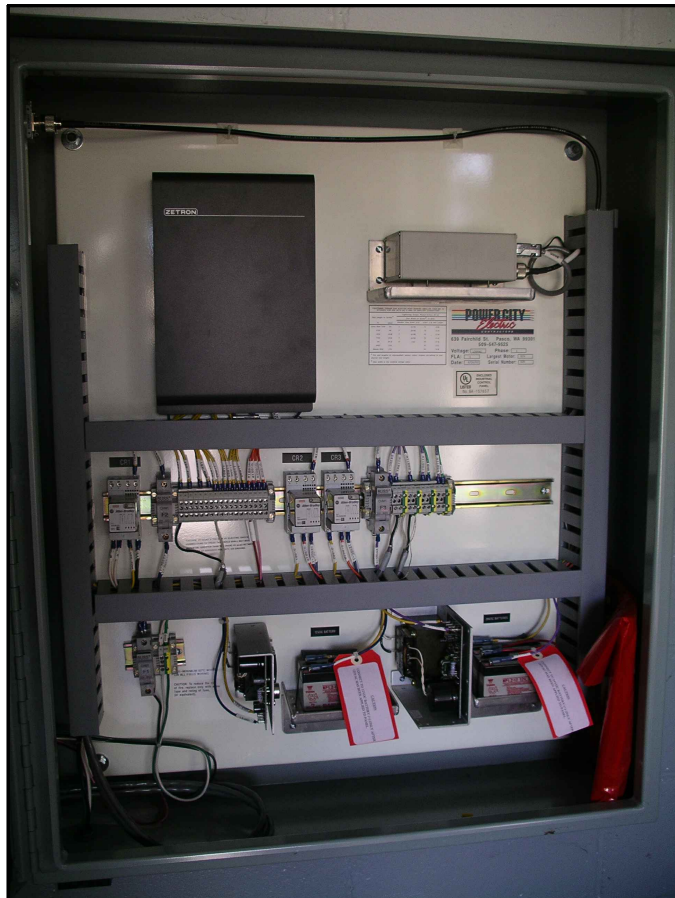
WELL HOUSE NO 2 TELEMETRY PANEL
