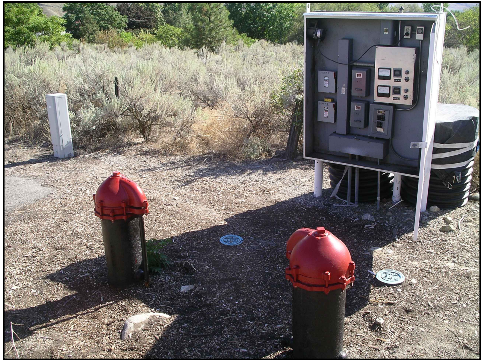
MURRAY STREET BPS (ELECTRICAL PANEL OPEN)
