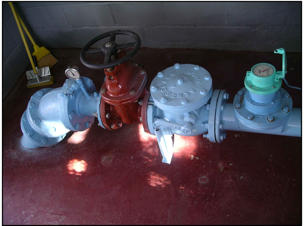
WELL HOUSE NO 2 VALVES & METERS
