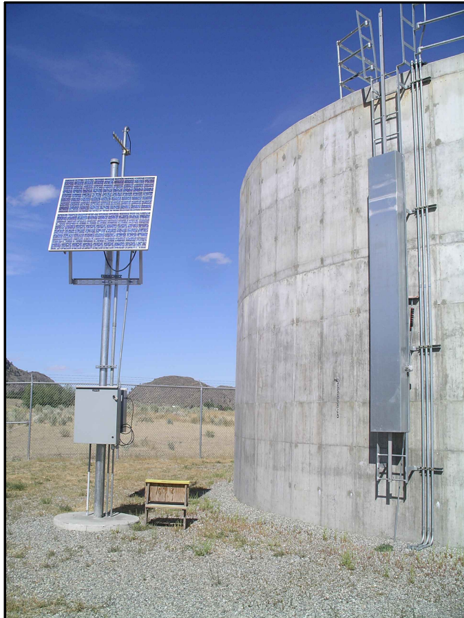
HIGHLANDS RESERVOIR TELEMETRY PANEL & LADDER ACCESS
