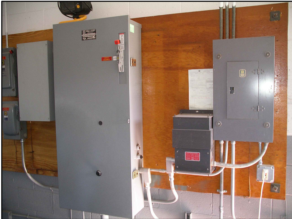
WELL HOUSE NO 3 ELECTRICAL PANEL
