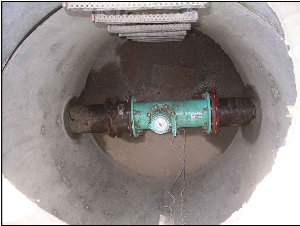
NORTH RESERVOIR BPS FLOW METER (IN VAULT)
