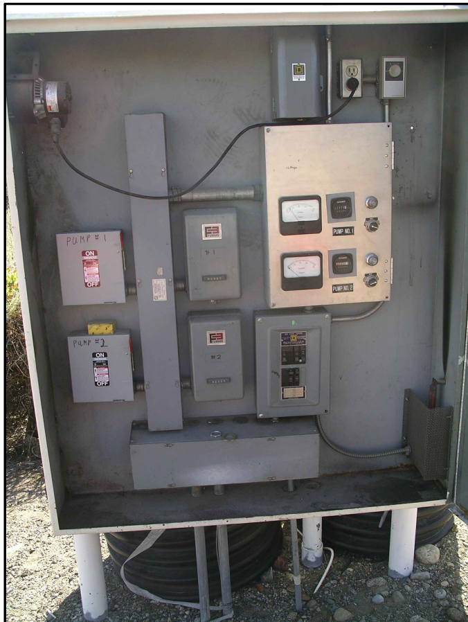
MURRAY STREET BPS ELECTRICAL PANEL
