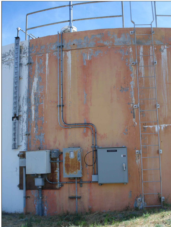
EAST RESERVOIR ELECTRICAL, TELEMETRY PANELS AND WATER LEVEL INDICATOR
