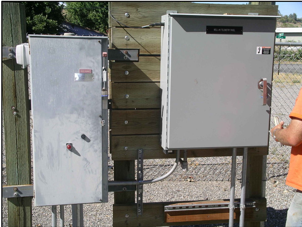
WELL NO 5 TELEMETRY PANEL
