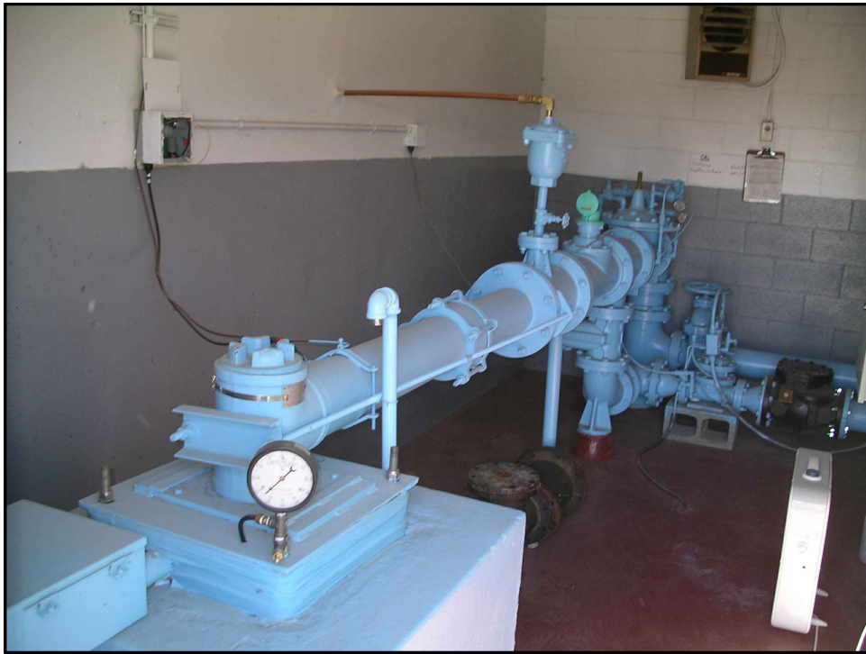
WELL HOUSE NO 3
