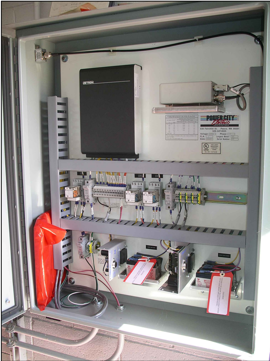
WELL HOUSE NO 3 TELEMETRY PANEL
