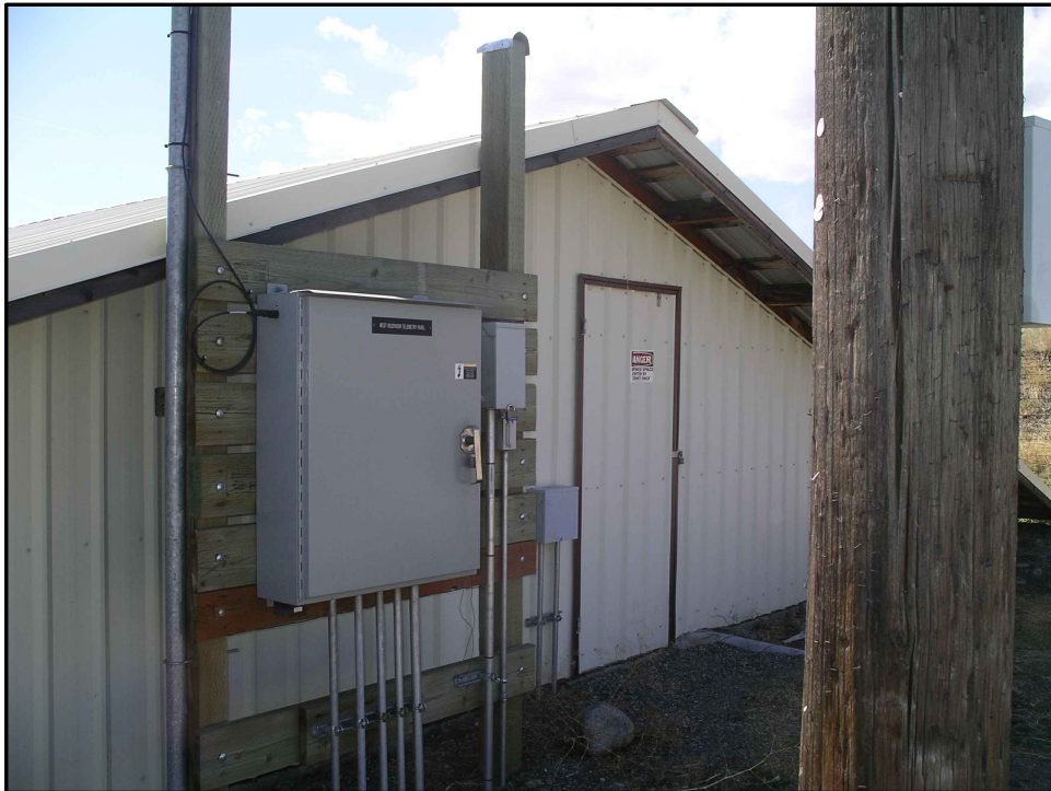
WEST RESERVOIR NO. 1 TELEMETRY PANEL
