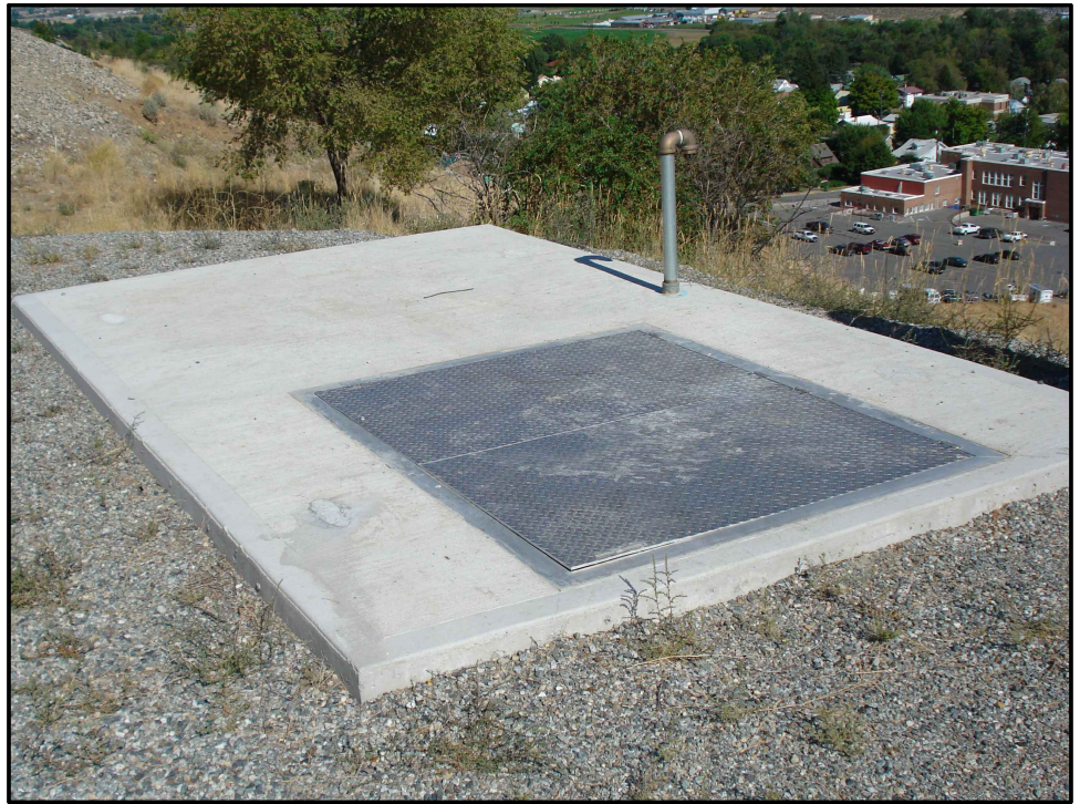
WEST RESERVOIR NO. 2 VALVE VAULT
