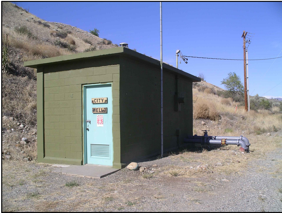
WELL HOUSE NO 3
